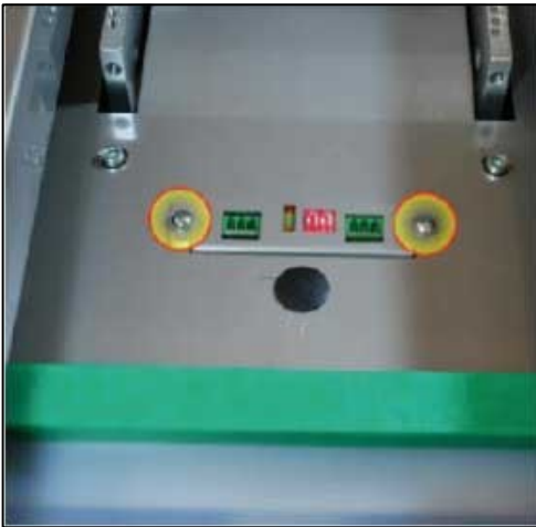
Figure 7-5: LED Controller (installed)
